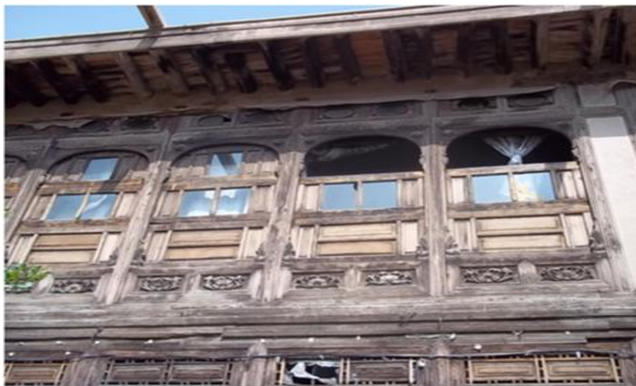
Fig.3 -general picture of the sashes of the peacock house with carvings (view from the side of the yard)
