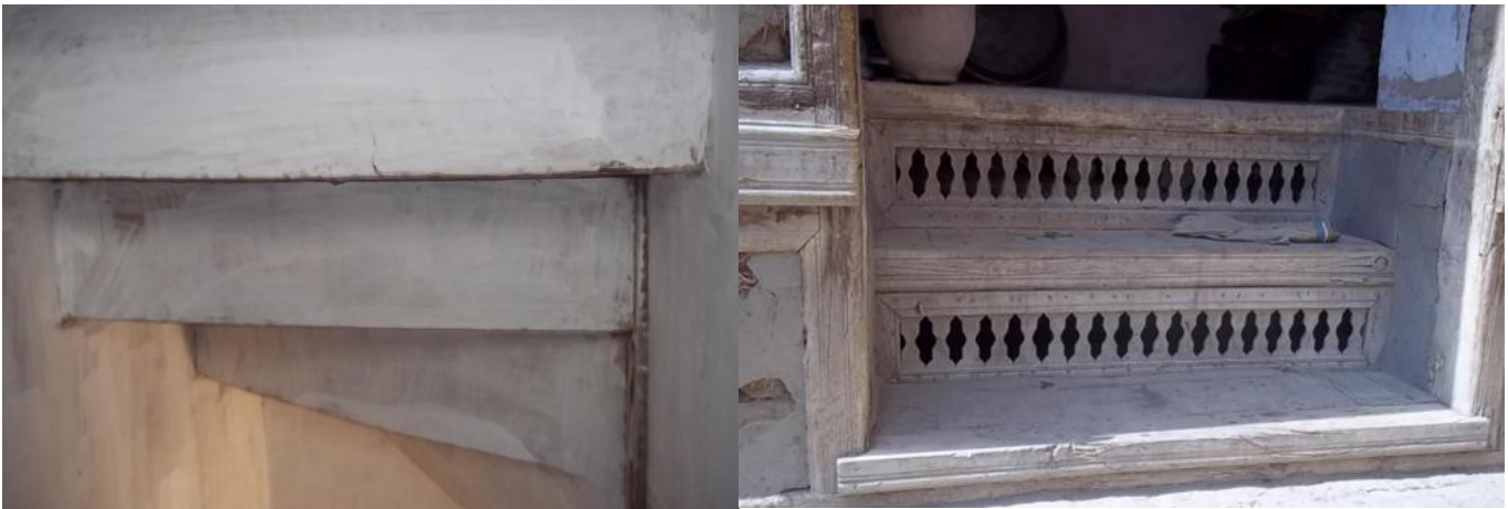
Fig.7 - Use of wood in the corner under the riser of the wooden stair (back view) and photo of a Kabul net in the rise of the wooden boards with very beautiful, airy and bright decorations (outdoor steps)
