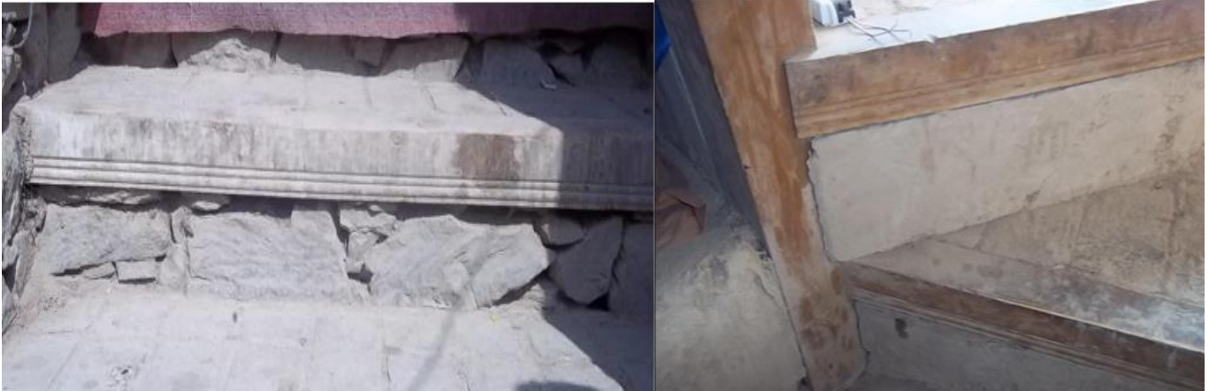
Fig.6 – Use of wood in the corner of the first and second steps of first floor and an images of the use of wood in the corner of the staircase (front view)
