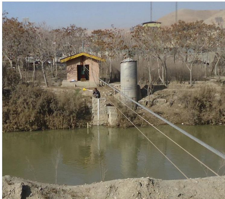
Figure 3. Stream Gauge Station at Tang-I-Gharu 1
