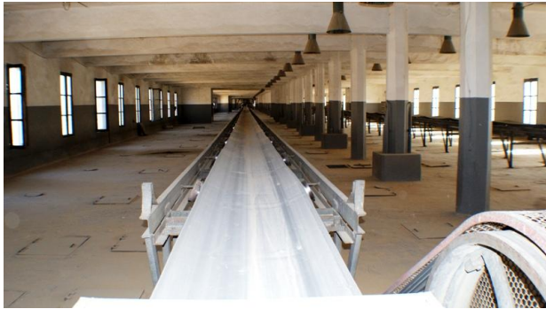
Kabul Silo Conveyers in need of replacement
