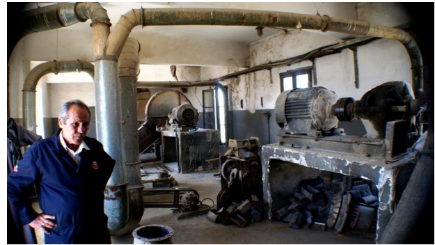
Kabul Silo: Equipment and duct pipes are broken.
